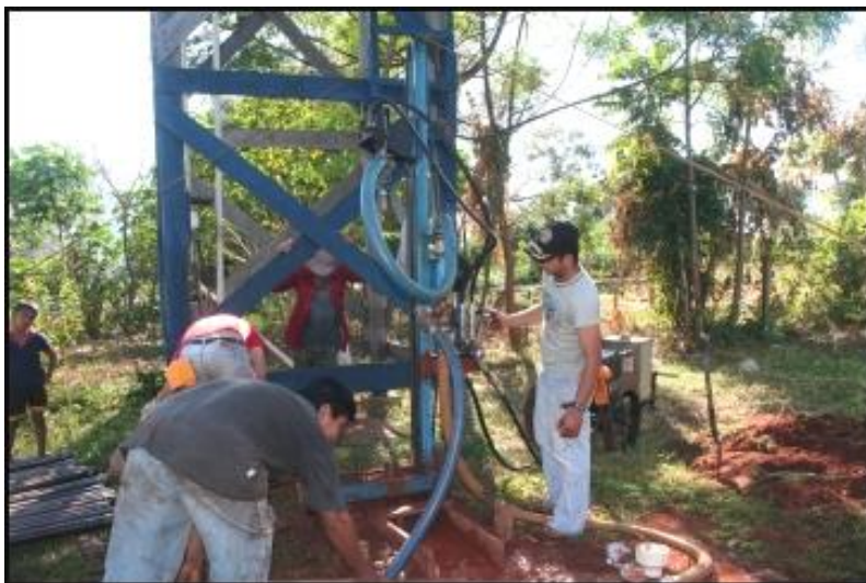
Well sites can be very messy! The new well is just in front of the old well and blue tower.
