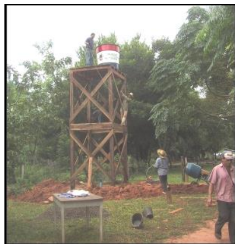
New tower and tank
